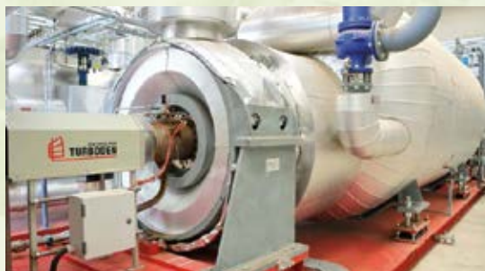
A typical Turboden ORC turbine and condenser arrangement.
